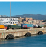
Pneumatic Fenders with chain & tire nets Ferry Terminal Ponto Colombo T7 Genova, Italy (2016)
