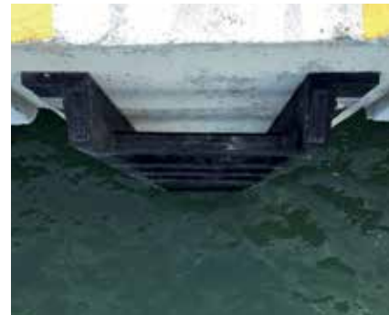
Feed Solid Product Jetty | Johor | Malaysia
