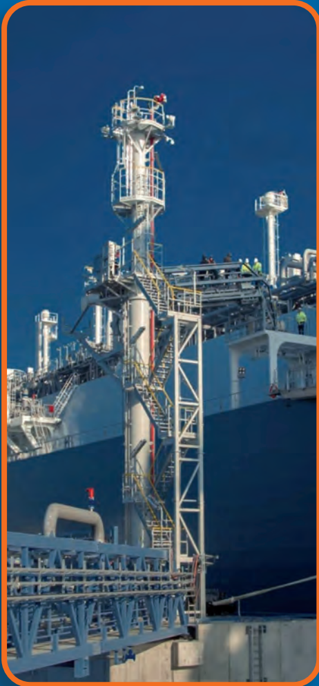
Column with fire monitor support on top. The telescopic gangway provides support for the ship-to-shore power supply. Klaipėdos – Lithuania.
